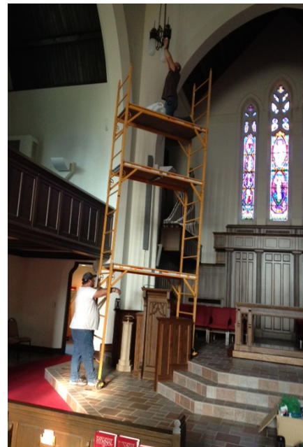
Workmen climbed up scaffolding to the top of the Sanctuary to install new light bulbs.
